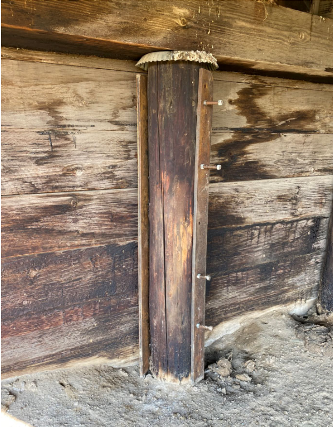
Picture 2 – Abutment pile split repaired with grader blades
